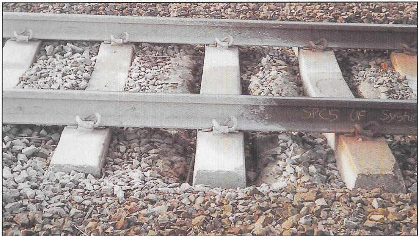
Voids: Water under pressure washes out ballast
