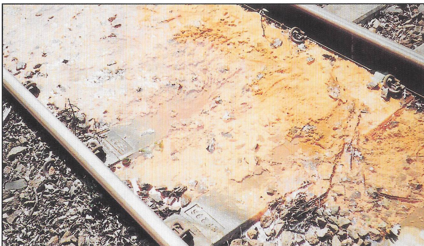
Contamination after flooding which if not cleared will lead to drainage failure
