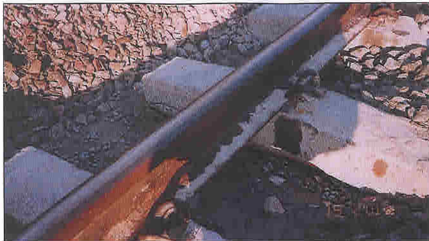
Wet Bed Site: Ballast removed to allow "Drying Out". This causes track distortion or buckling in hot weather
