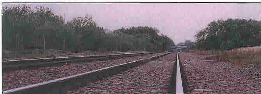
Typical top fault on wet bed site showing a single irregularity
