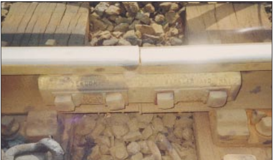
Figure 1 Lipping of the rail ends due to normal traffic.
