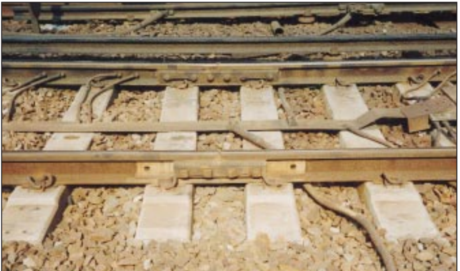
Figure 9 6-Hole prefabricated joint replaced using a 4-Hole Benkler The above practice should only be used as a temporary repair. The increased flexibility in the 4 hole joint in relation to 6 hole may lead to the generation of a twist.
