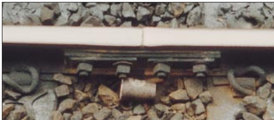
Figure 5 failure of fish-plate shells / liners - insulation's
