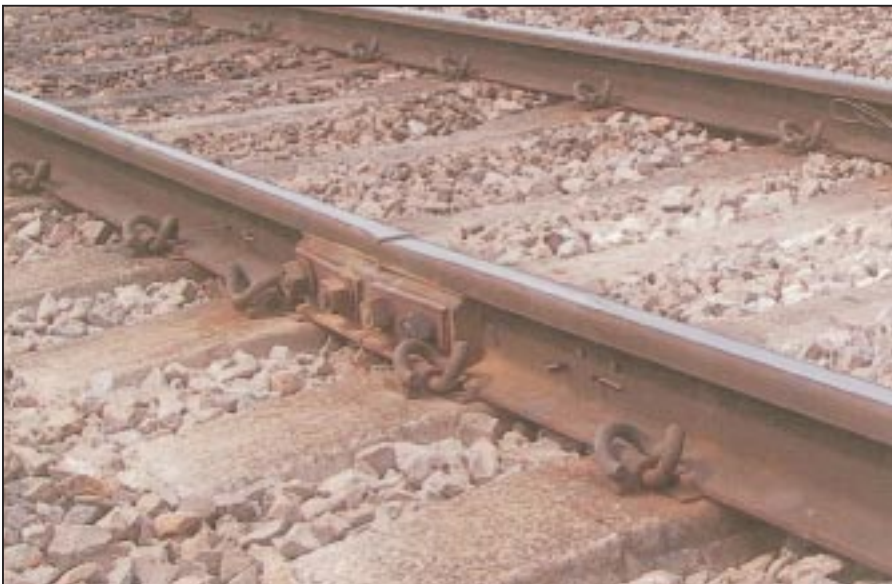
Figure 8 Treble Six Nylon Joint (In a poor condition).
