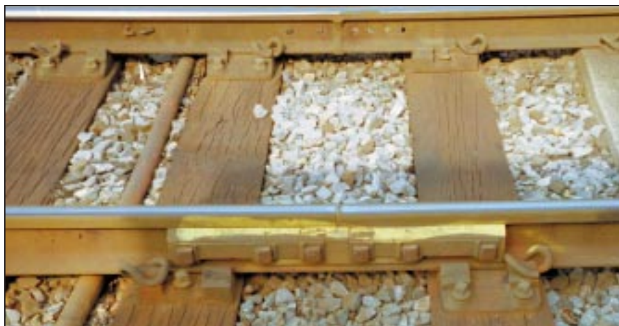
Figure 6 Incorrect sleeper spacings, note that the spare housings look correctly positioned. Pan 14 baseplates would alleviate this problem.
