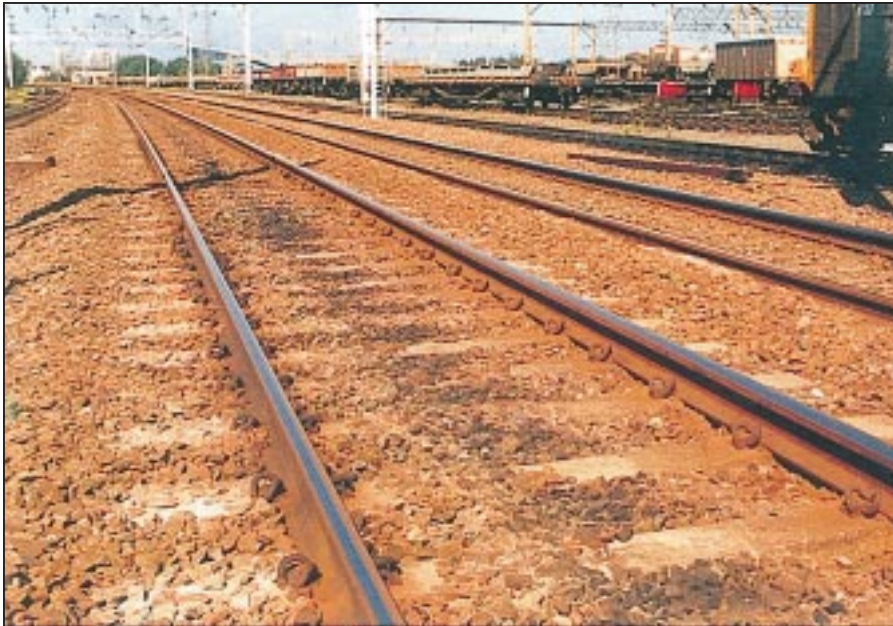
Photograph - Lighter coloured ballast on the sleeper ends indicates voiding.
