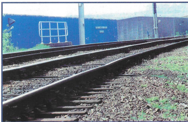
Badly Dipped Joints On Wooden Sleepers
