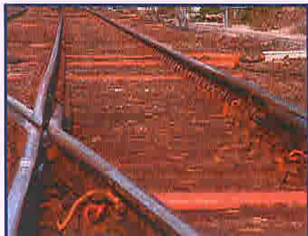
Less severe misalignment on left hand rail just off the crossing nose
