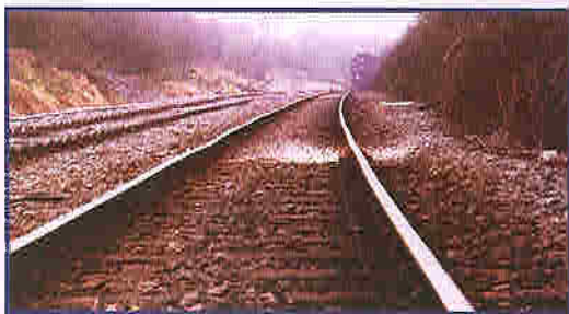
Poor Top in Jointed Track
