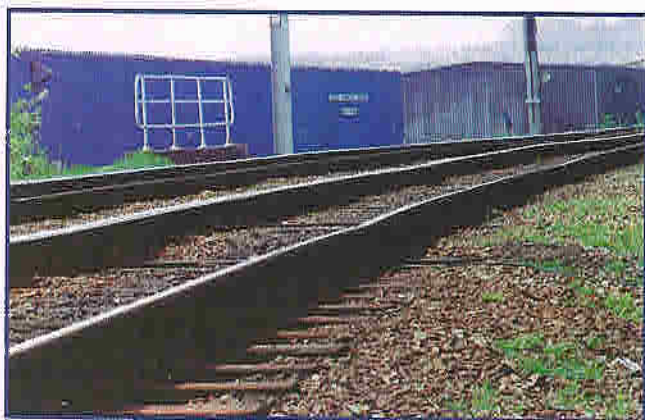
Badly Dipped Joints On Wooden Sleepers
