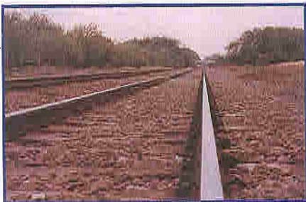
Typical area where wet beds have been allowed to develop to a stage where twist has now become a problem.
