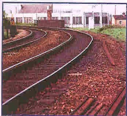
Dipped and poorly aligned joints together with generally poor longitudinal profile of the right hand high rail combine to produce a poor quality railway
