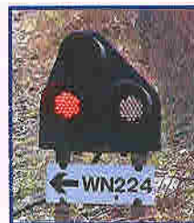
A ground signal to allow for controlling trains out of sidings on to a main line
