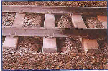
No Subgrade layer has been installed and conditions deteriorate
