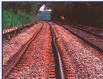
Misalignment provides a trigger point for track buckles
