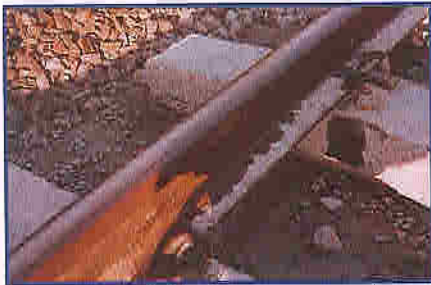
The Wet bed has developed to a point where if the ballast was removed it could result in buckling/distortion of the track.
