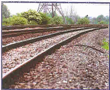
Poor Top In Continuous Welded Rail(CWR) On Concrete Sleepers
