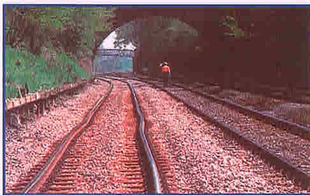
In the picture above we can see the result of hot weather on incorrectly maintained track - in this case poorly installed ballasted steel sleepers.
