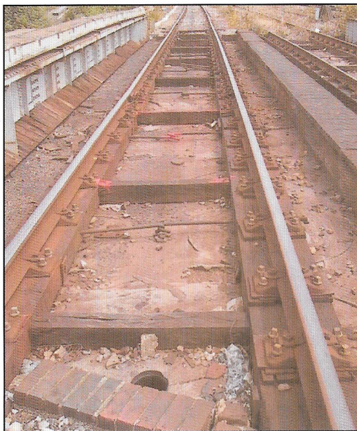
Figure 7 A typical longitudinal timber bridge. Once again the packings used do not cover the baseplate foot print area, note also how close the screw hole centres are to the edge of the timbers.
