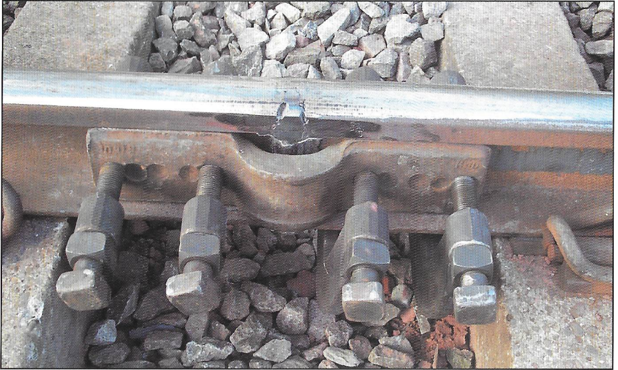
Fig 4. G-Clamps used with joggled plates to protect a defective weld.
