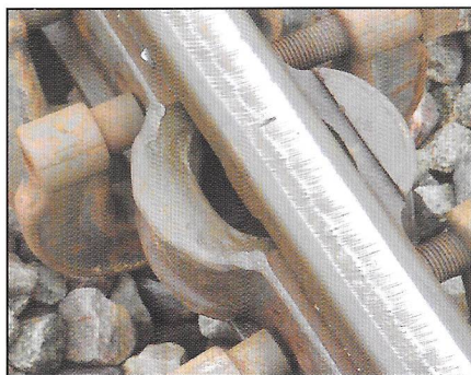
Emergency Fishplates fitted incorrectly on site. (Left hand plate is upside down)
