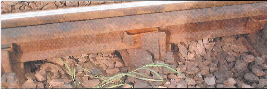
John Bradley Bullhead Keys inserted incorrectly into a check rail
