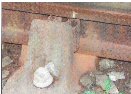
An incorrectly installed Tapered Steel Bullhead Key
