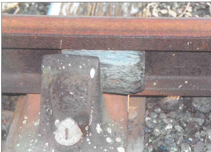
A wooden Bullhead key in poor condition providing insufficient hold on the rail
