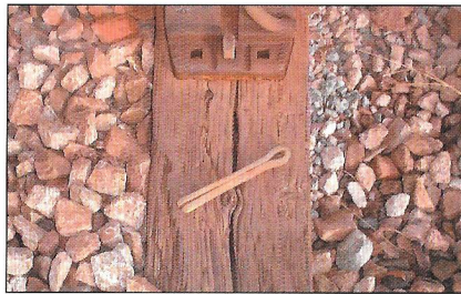
A severely corroded Lock Spike removed from a baseplate. (Note the normal appearance of the head of the spike)
