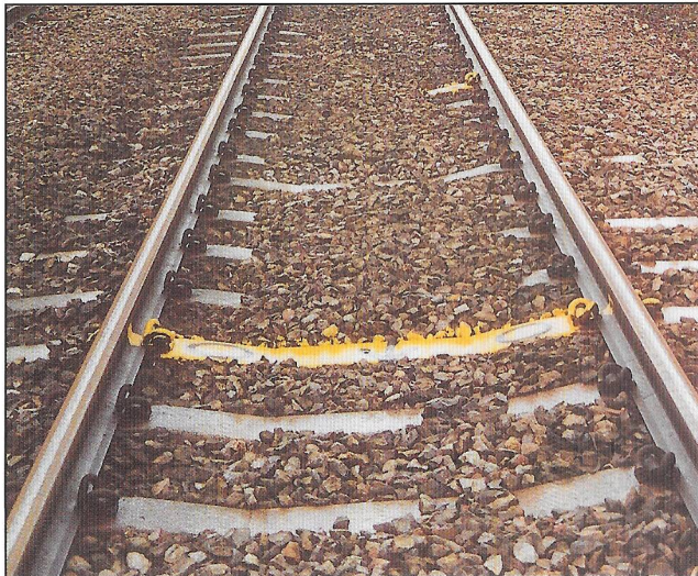
Photograph- transition curve with cant marking
