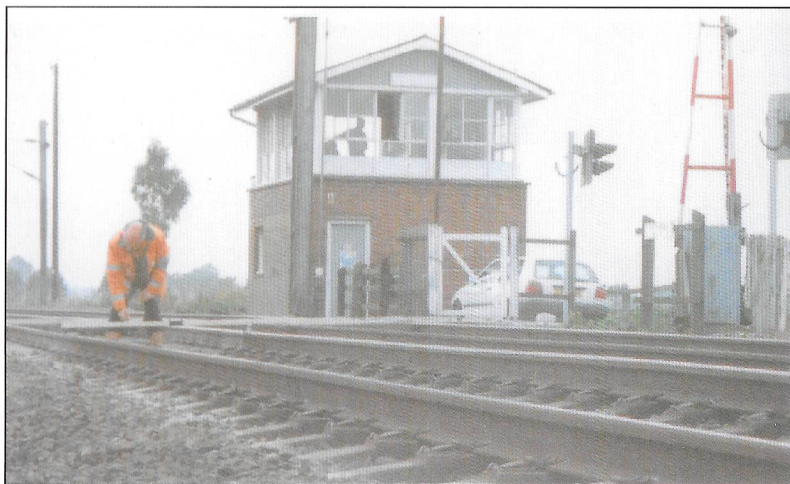
Photograph - twist fault measured at a Level Crossing
