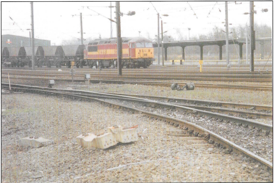
Photograph - derailment risk twist fault in S&C
