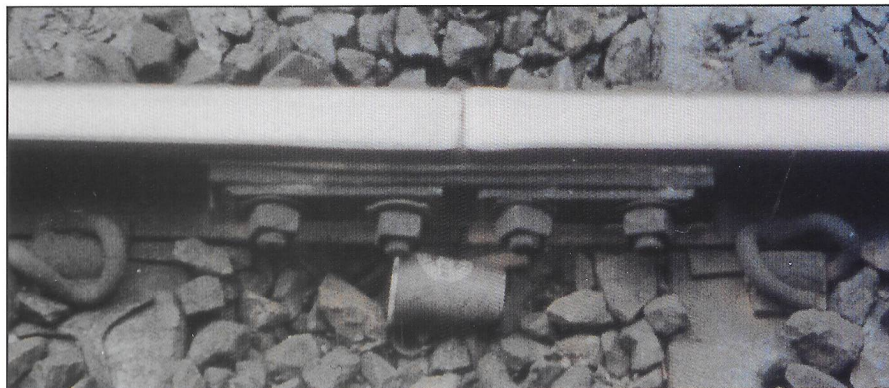
Figure 5 failure of fish-plate shells / liners - insulation's
