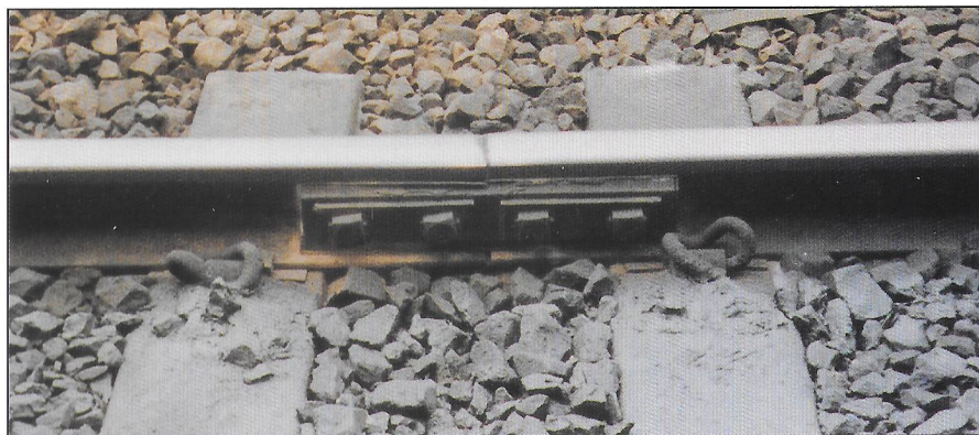
Figure 2 'T Piece' (End Post) Broken and damaged insulation.
