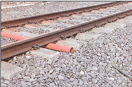
The sleeper ends are exposed, so there is inadequate horizontal shoulder ballast, nor is it piled 125mm high.
