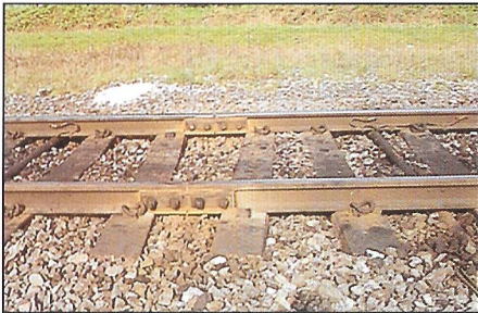
The sleepers are out of square, fastenings are missing and the insulated joint, appears to be breaking up.
