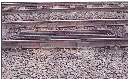
Some voiding of this adjustment switch is apparent from the white dust on the sleepers and baseplates.
