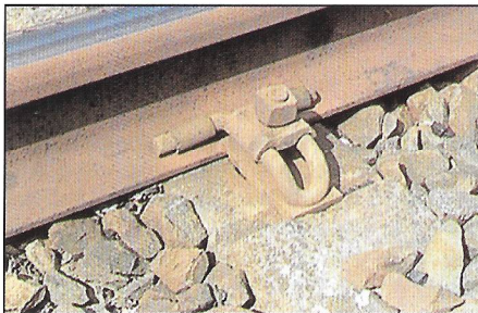
A maintenance screw has been fitted to this BJB fastening, but the gauge plate is on top of the rail foot, so the gauge is suspect.
