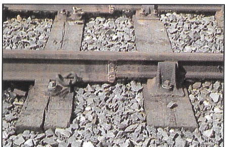
A composite weld at the change from flat bottom to bullhead rail.
