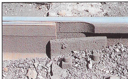
Both these adjustment switches require urgent attention.
