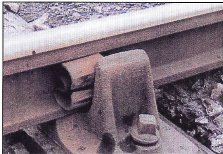
This steel key does not fit correctly. The ballast is very dirty.
