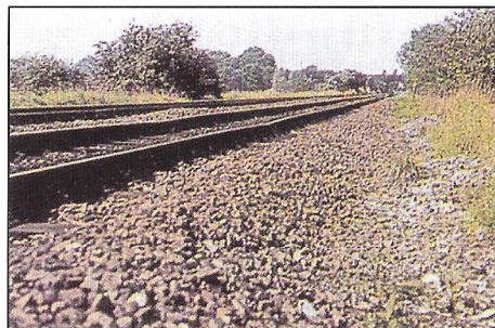
Dipped joints such as this will cause the rails to be driven forward.
