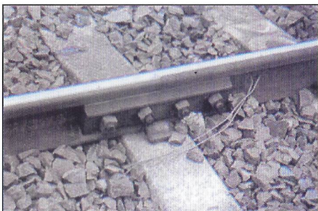
A joint on top of the sleeper. When was it last lubricated or pulled back?
