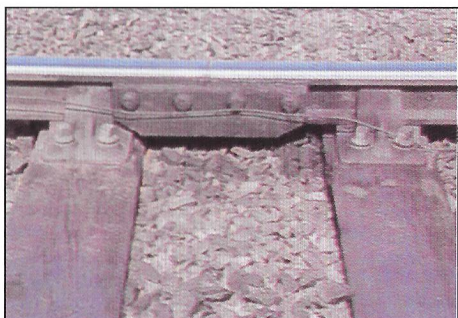
This BH fishplate has been driven hard against the chair by the creep.
