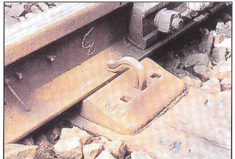
This spike is ineffective; the rail is not tight in the baseplate and the baseplate is shuffling.
