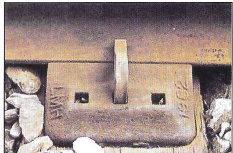
The marks on the top of the rail foot, to the left of the spike and to the right of the baseplate indicate that the rail has been pulled back at least twice.
