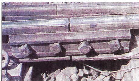
The heel joint at a cast AMS crossing. No TJ plates and a mixture of bolts, permitting the plain rails to move.
